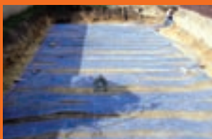
Laying of a space-saving NIBE compact absorber as effective energy source in the garden
